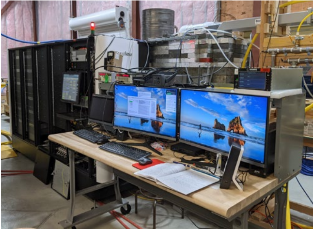
Fig. 3. A test station used for testing a modulator, Klystron and RF windows.
